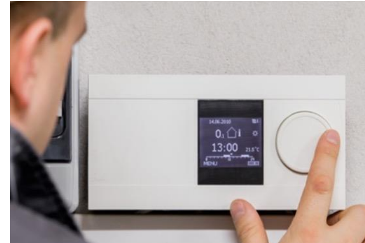
Implementing energy efficient building controls
