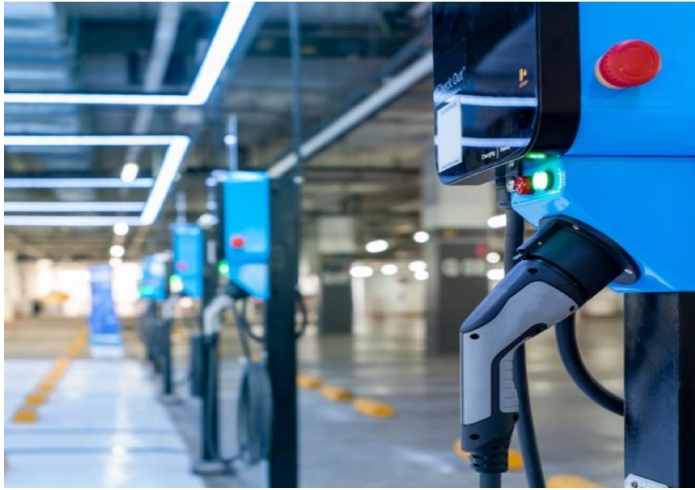
Locating EV chargers throughout RSC
